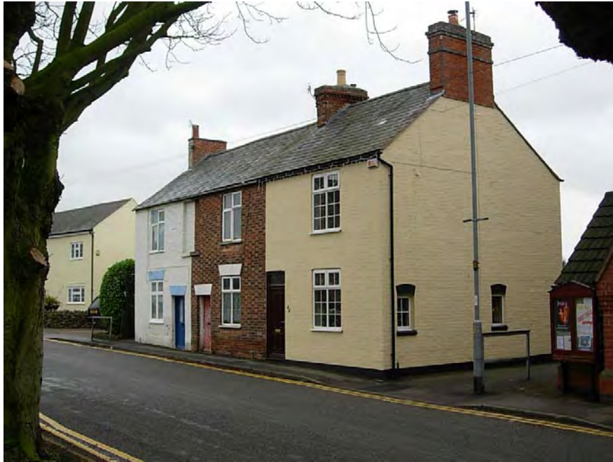
44 – 48 Main Street is a pleasant terrace that has lost its unity with new plastic windows inserted and two of the three properties painted/rendered.
