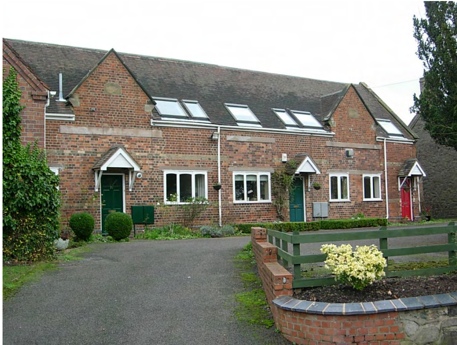
The former village primary school has lost some of its charm with the insensitive use of artificial materials and insertion of large roof lights on the street elevation.
