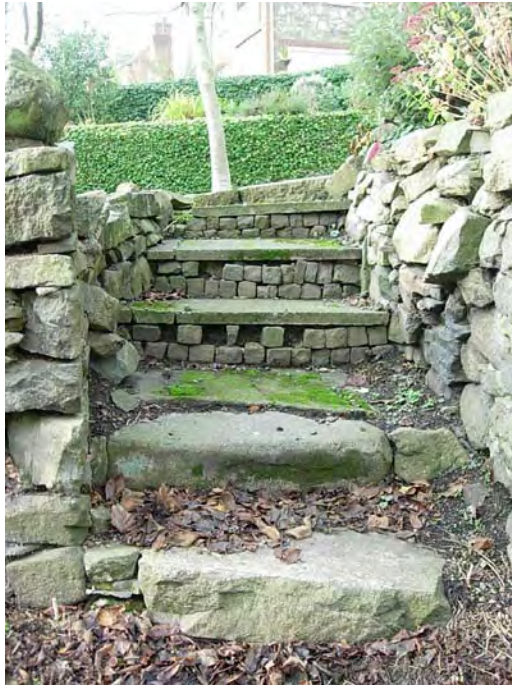
The steps leading up to 51 The Green are in need of maintenance.
