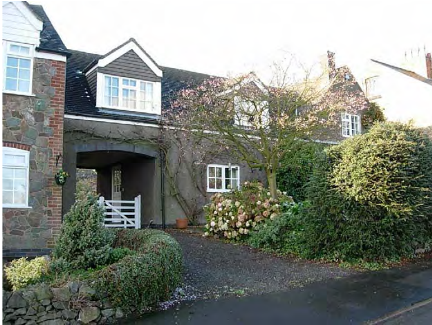
The dormers at 33 The Green are out of scale with the building fabric and the detailing does not follow the traditional form.
