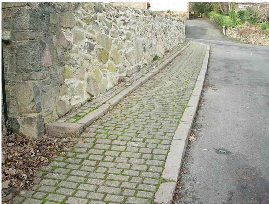
The use of granite setts to match the granite kerbs would have been preferable to the use of concrete paviours in this sensitive area fronting the parish church.
