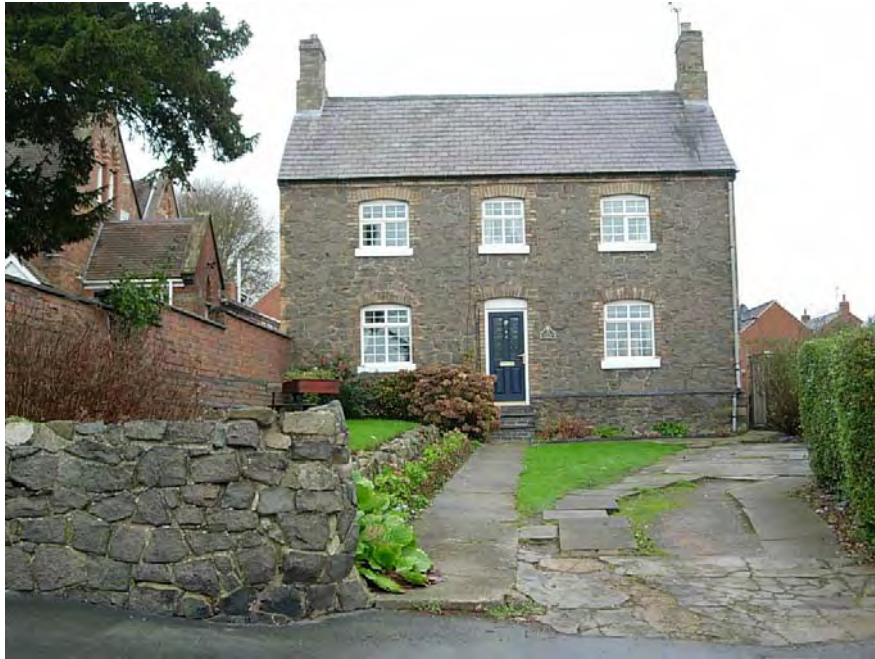
The Old School House, 10 The Green, is a fine granite dwelling with a slate roof and two chimney stacks but the car parking space fronting the property needs attention.
