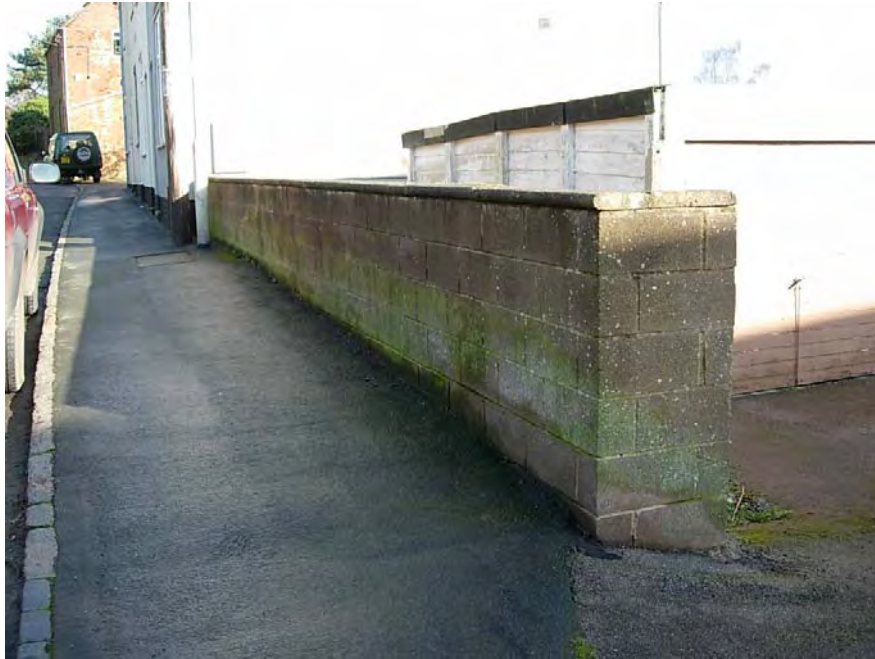
The concrete block wall fronting the garage court at 38 The Green needs replacing with a traditional granite wall.
