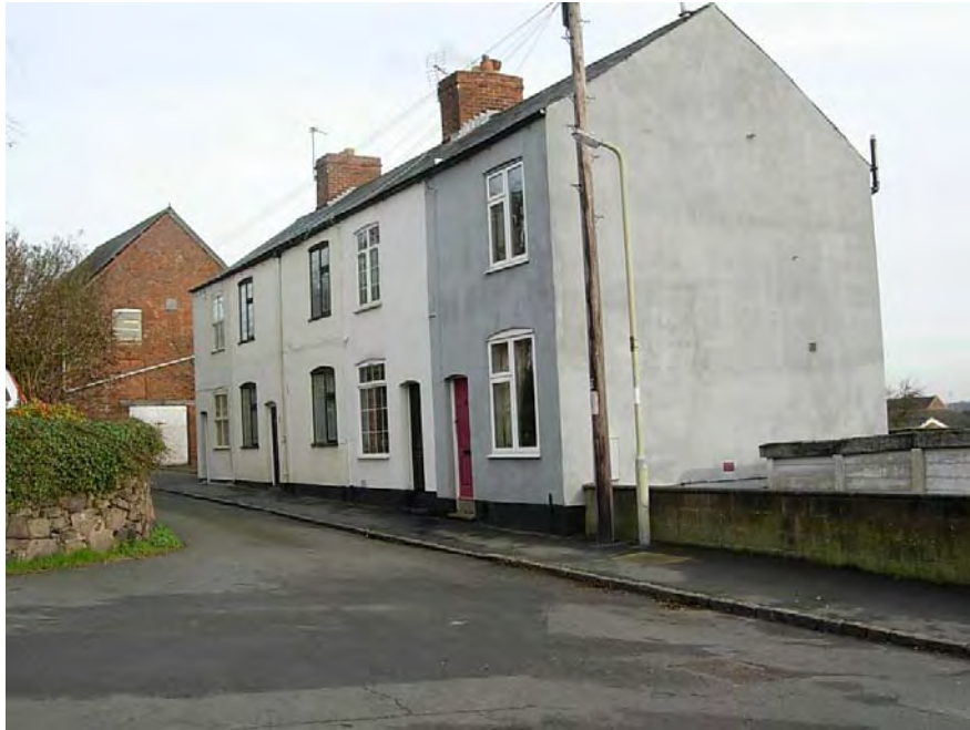
The introduction of modern replacement windows at 44 - 52 The Green has had a detrimental effect in this terrace.
