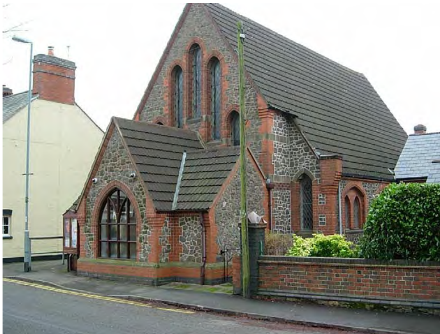
The Trinity Methodist Church is spoilt with the use of concrete tiles.
