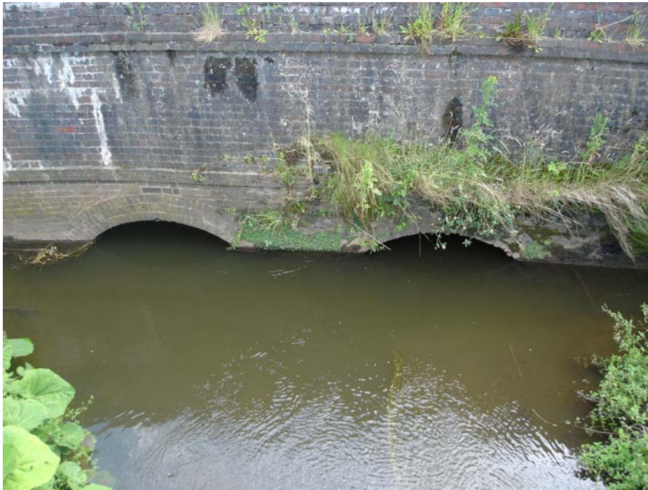
The River Sence passing under the Shackerstone aqueduct. The aqueduct is in need of some maintenance.
