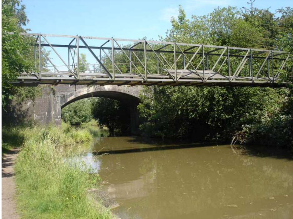
This unattractive large metal frame structure used to carry cables across the canal is particularly prominent. A more elegant replacement structure should be considered.
