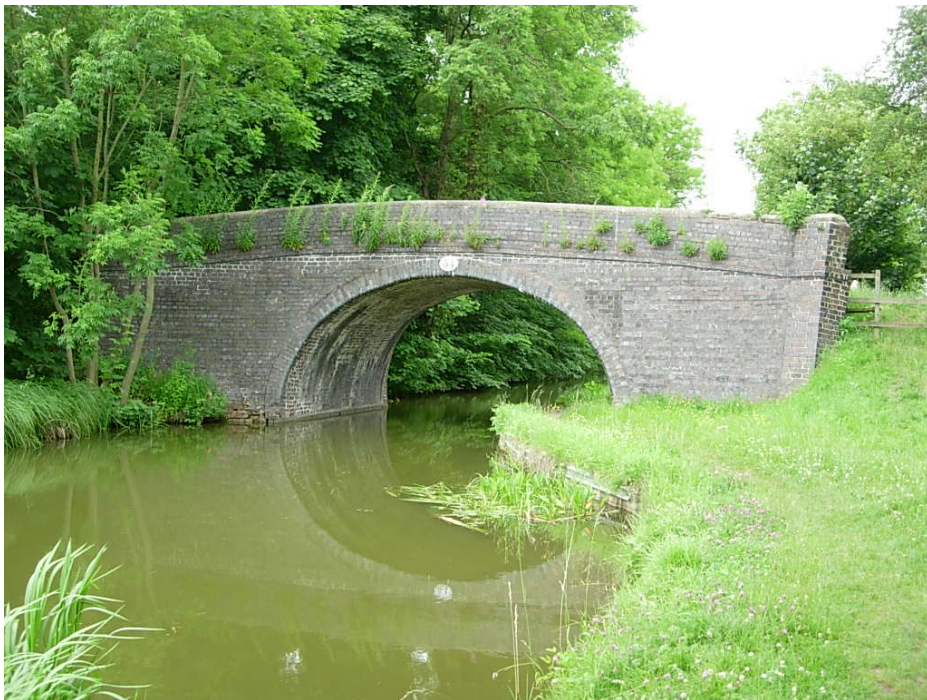
One of the numerous single arched bridges that span the canal generally built in blue or brindle blue bricks. The bridges are important features associated with the canal's industrial heritage that should be retained at all cost.
