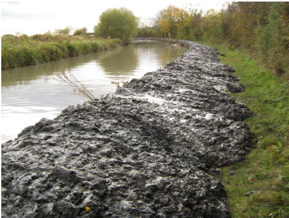
The current dredging of the canal and deposit of the sludge on the towpath is having a significant detrimental impact on walkers and the appearance of the canal. It is unacceptable and should be taken off site.
