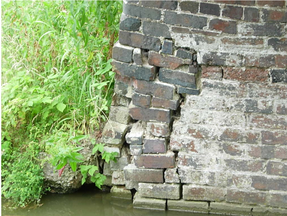
Bridge 31 is in a very dangerous state of repair and now requires partial demolition and re-building.
