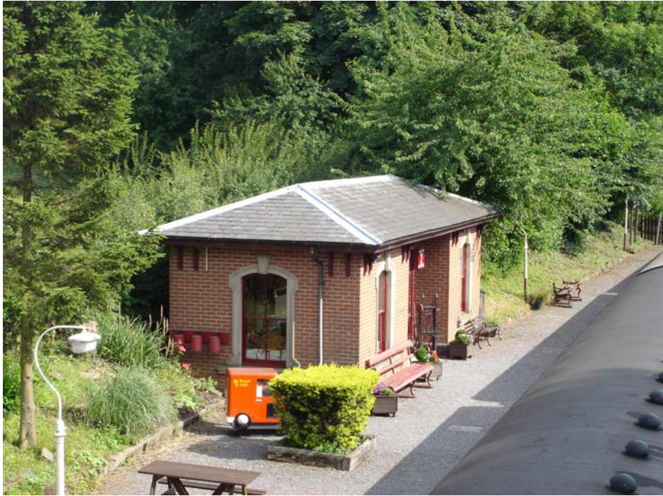
A non traditional brick bond has been used in the construction of this new building at Shackerstone Station and the pointing is overly prominent.
