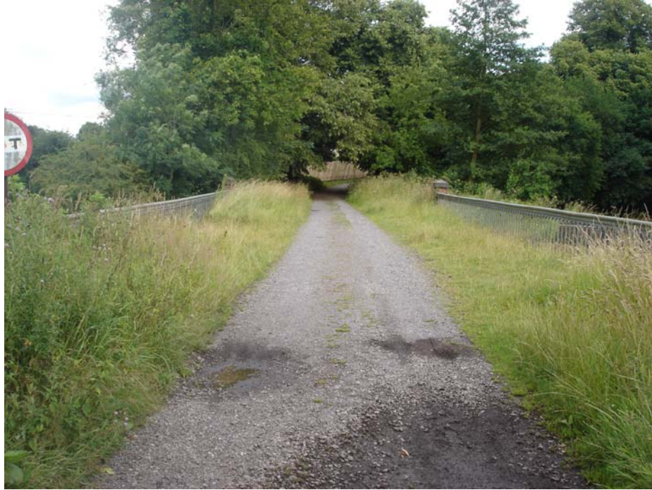
The track leading to Shackerstone Railway Station. The road bridge built around 1873 is a Grade 2 listed structure made of cast iron built on red brick supports with 3 bays spanning the River Sense. It has cast iron open parapets with brick end piers and stone caps .
