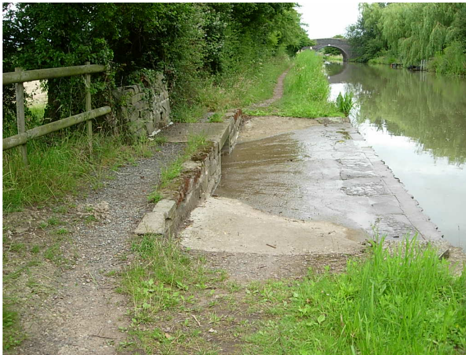
One of the overflow weirs on the Ashby Canal that drain into adjacent streams and ditches.
