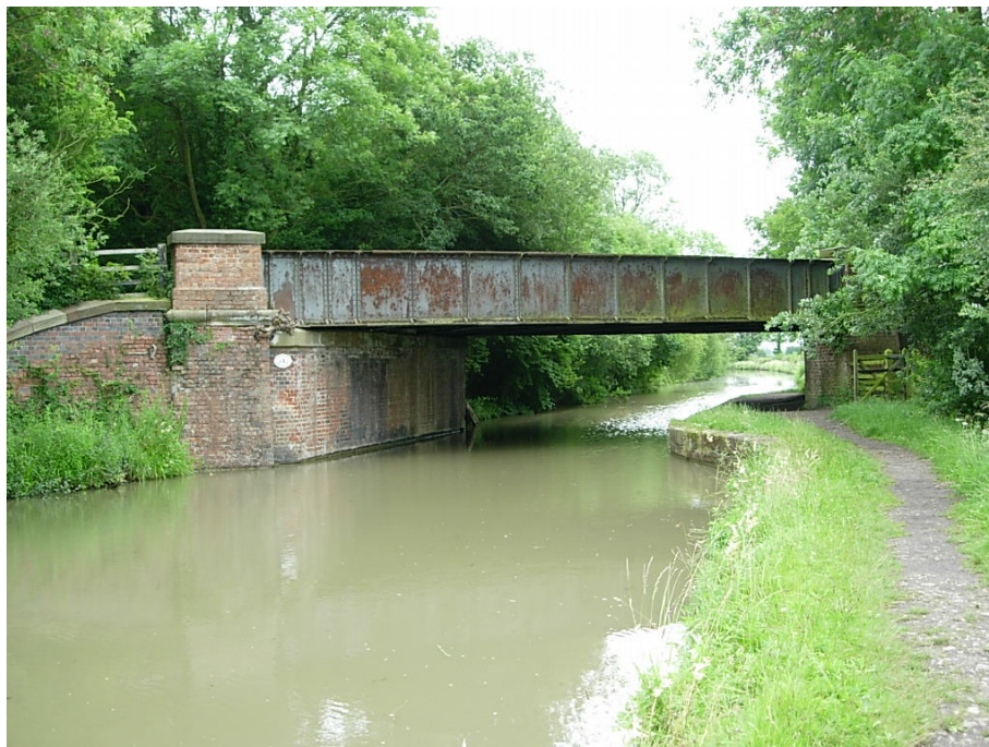
Bridge 34A that once formed part of the Ashby to Nuneaton branch railway line is now used by pedestrians. It is a fine steel structure that needs repairing and painting.
