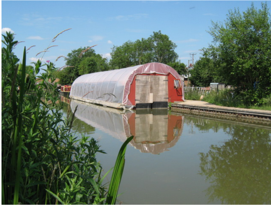
A temporary poly-tunnel used for boat repairs sited along part of the canal that has been sheet piled. Although an unattractive feature, it is needed for the viability of the canal as a tourist attraction.
