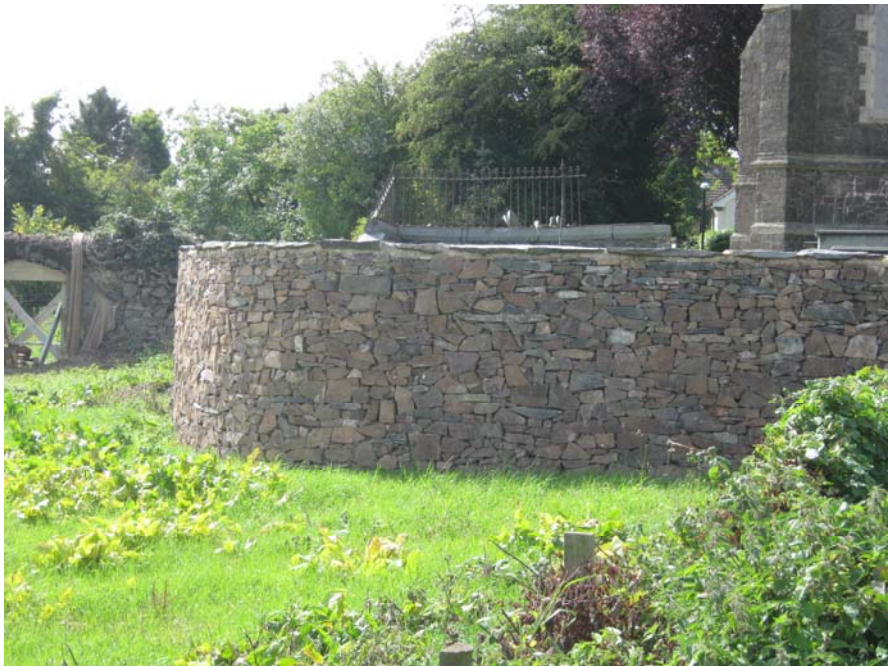
The churchyard wall has recently been re-built and is a good example of new stone construction.
