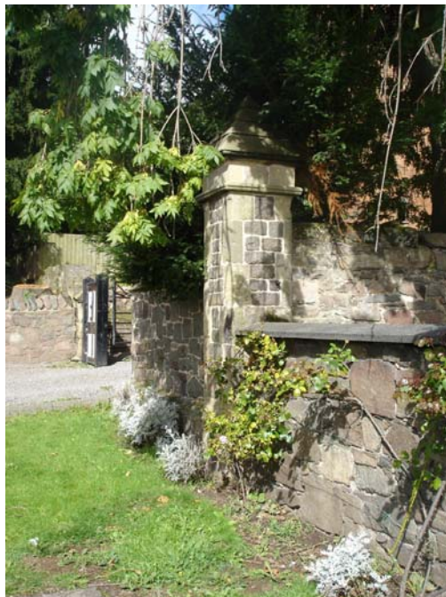
Stone pier fronting the Old Hall. The other pier on the western side of the access has been considerably reduced in height.
