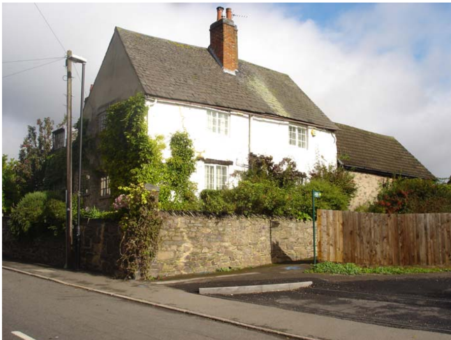
30 Markfield Road is a Grade II listed C16 timber framed property that has been overbuilt in Mountsorrel granite and colour washed. Unfortunately, the adjoining building has been re-roofed with concrete tiles. These should be replaced with natural slate in the long term.
