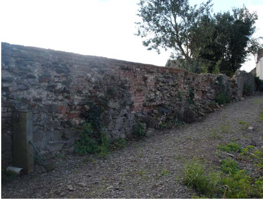
This wall sited in the allotment gardens on Markfield Road is believed to be part of the Old Hall's gardens. However, it should be retained and needs repairing.
