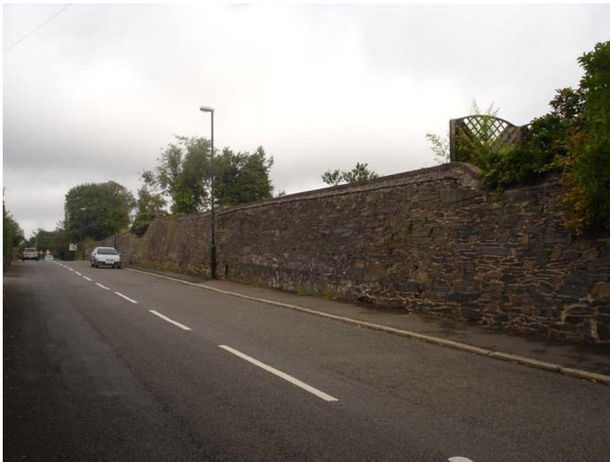
The excellent stone retaining wall runs up the north side of Markfield Road flanking one of the village's allotment gardens. It is a key feature in the conservation area.
