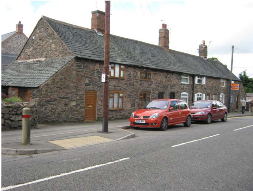
The unity of this terrace of stone properties on Leicester Road has been compromised by the inappropriate modernisation of its windows, doors and loss of some chimney pots.
