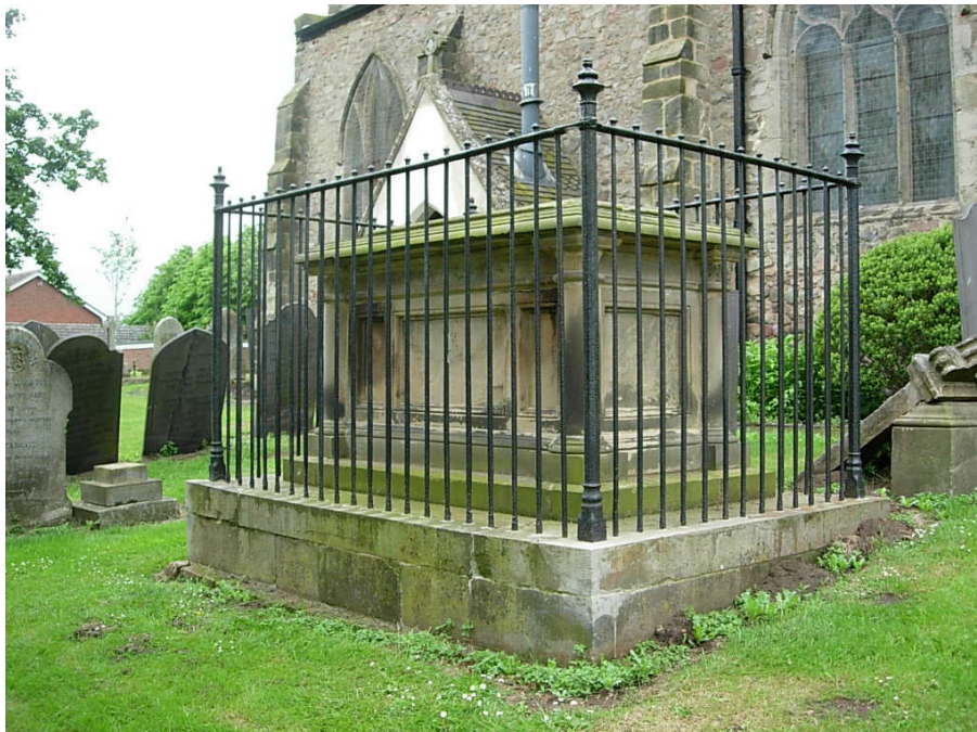
The chest tomb today. These tombs are important historic and architectural features that will be lost to future generations unless they are restored.
